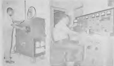
At left, Area Supervisor Arnold Beyde tries out new circuit breaker testing unit, while at right Acting Area Supervisor Harry Koolman is with the frequency generator at the relay test table.
